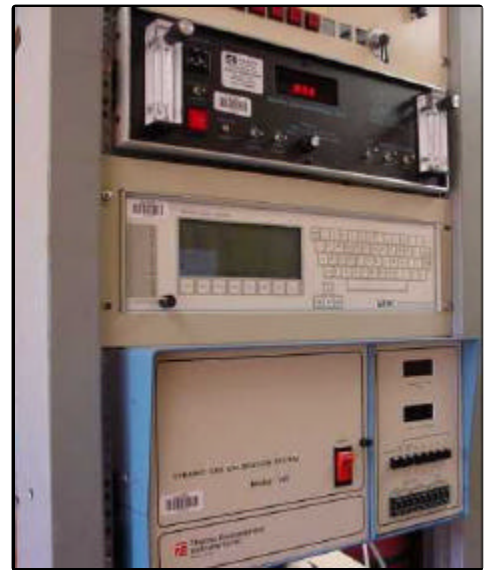
Figure 2: Continuous Monitoring Equipment located within an Air Monitoring Trailer
